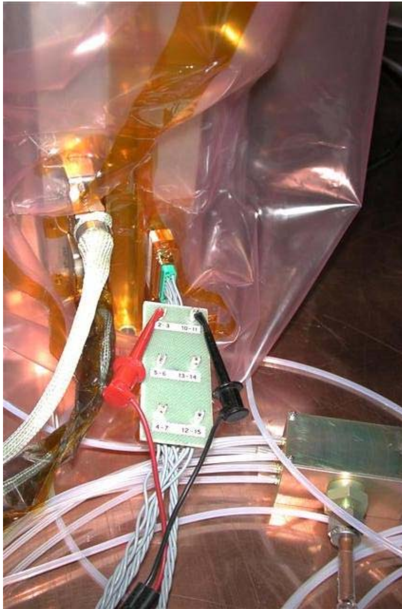
Figure 10-4. Close-up of the CS06 Connection to Stereo Impact Input Power Leads
